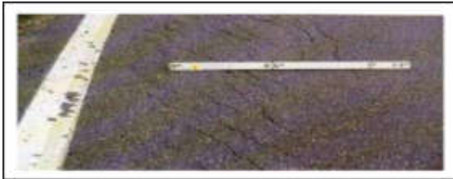
Gambar 2.38 Patah Slip ( Slippage Cracking )
