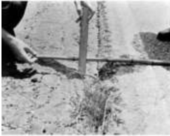
Gambar 2.22 Pinggiran Jalan Turun ( Lane/shoulder Drop Off )
