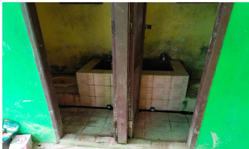
Gambar 4.2 WC/Jamban SMA Agape Tanjung Selor
