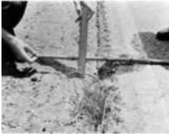
Gambar 2.22 Pinggiran Jalan Turun ( Lane/shoulder Drop Off )
