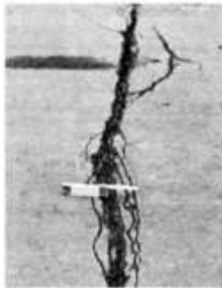
Gambar 2.20 Retak Sambung ( Joint Reflect Cracking )
