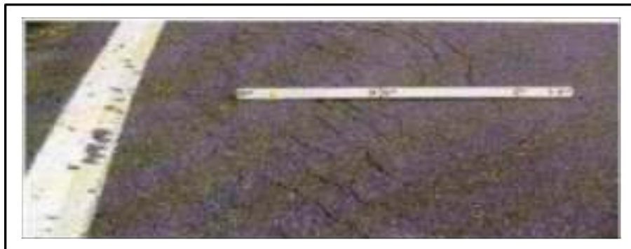
Gambar 2.38 Patah Slip ( Slippage Cracking )
